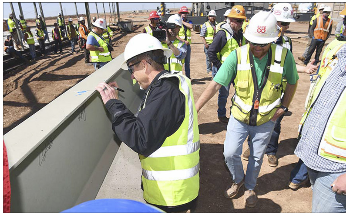
Workers sign the last beam to be placed on the new High Explosives Science & Engineering facility at the Pantex plant last week.
