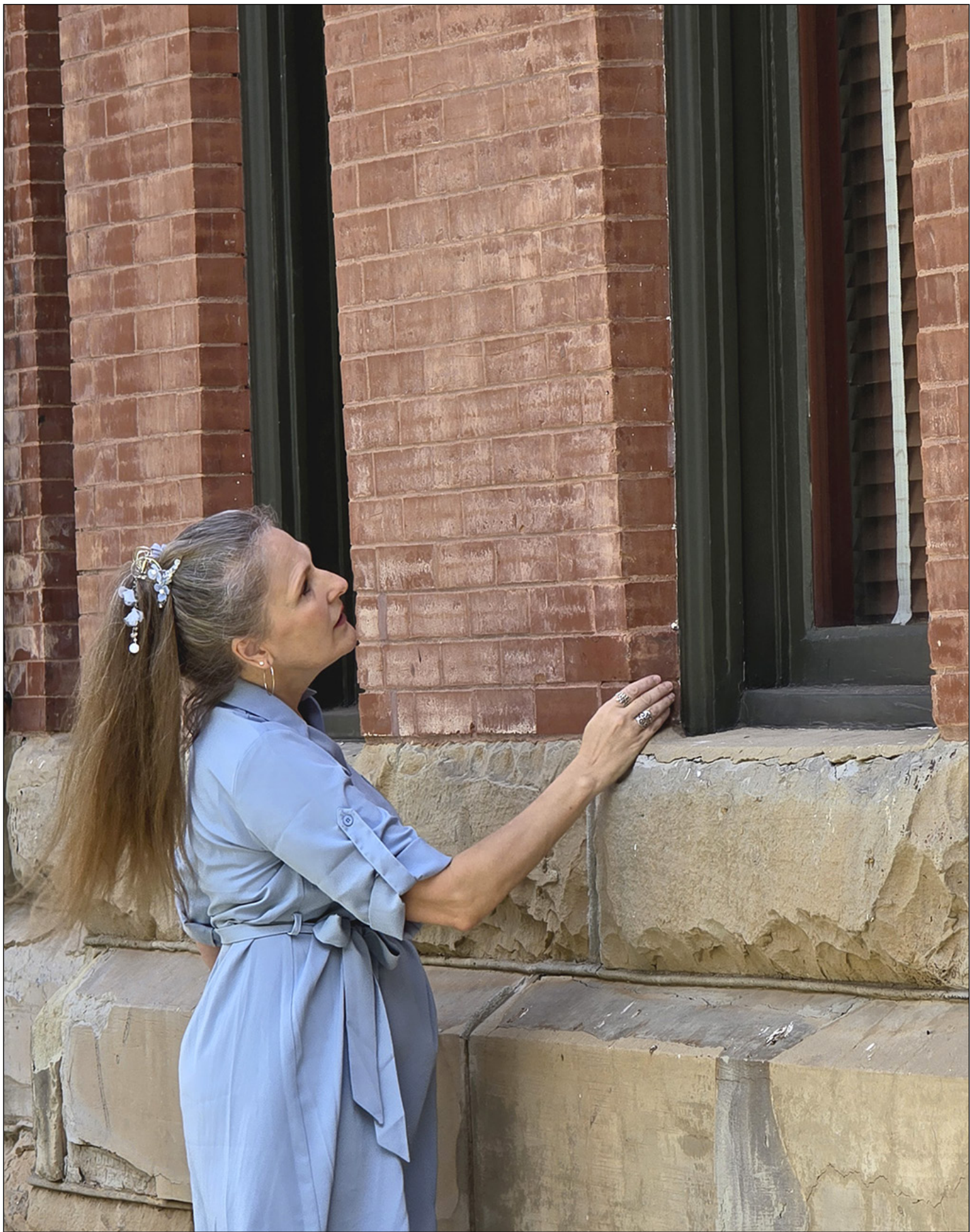
Architect Tracy Hirschman Hutson examines a section of facing brick that is bulging on the south side of the Donley County Courthouse during a visit here on Monday. Following up from her right hand, it is visible how the brick has moved out over time.
